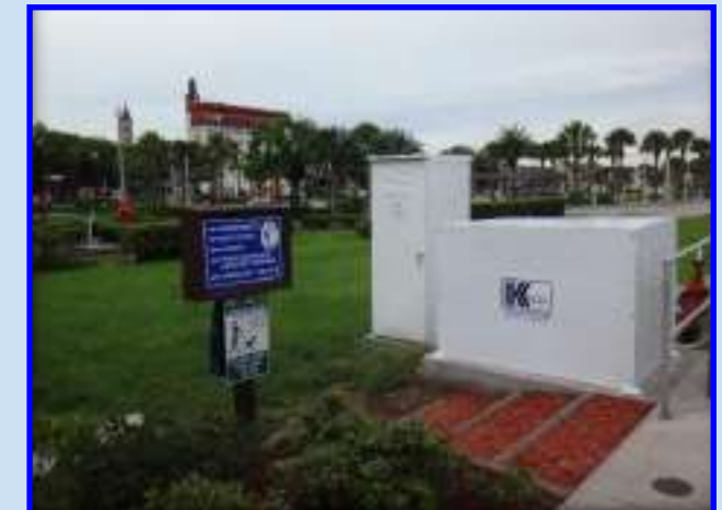
These photographs show examples of stationary sewage pump out facilities. These are located (from left to right) at City of Hallandale Beach, Mariner Cay in Martin County, Titusville and Saint Augustine.
