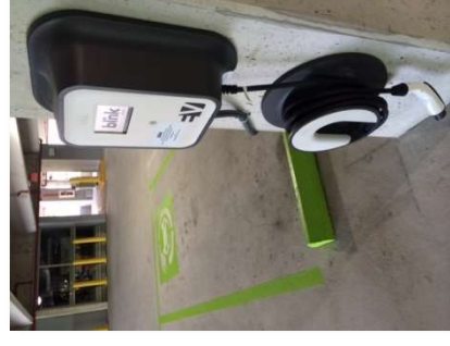
Blink charging station in City Hall Parking Garage.
