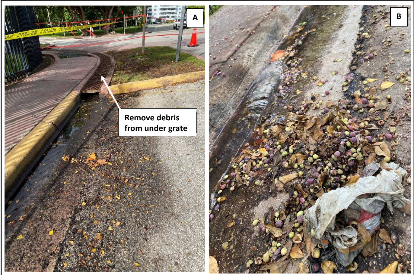
Figure B.2. The storm drain grates at most corners (Panel A) should be lifted and debris removed as part of regular street sweeping. Debris left behind by street sweepers at the end of the run should be picked up manually (Panel B).
